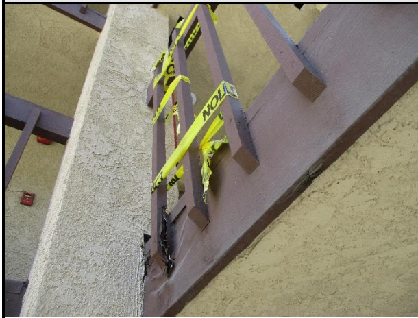
Picket and Fascia Deterioration
