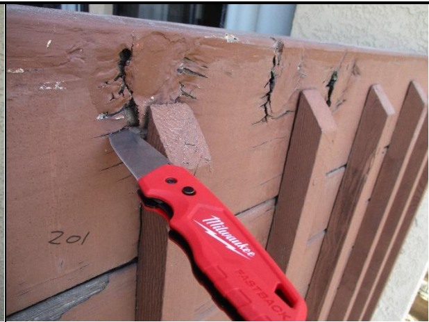
Balcony with Rotten Handrail
