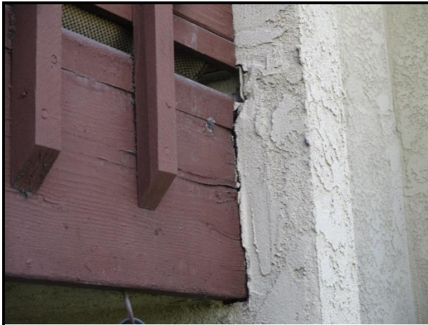
Balcony with Poor End Flashing
