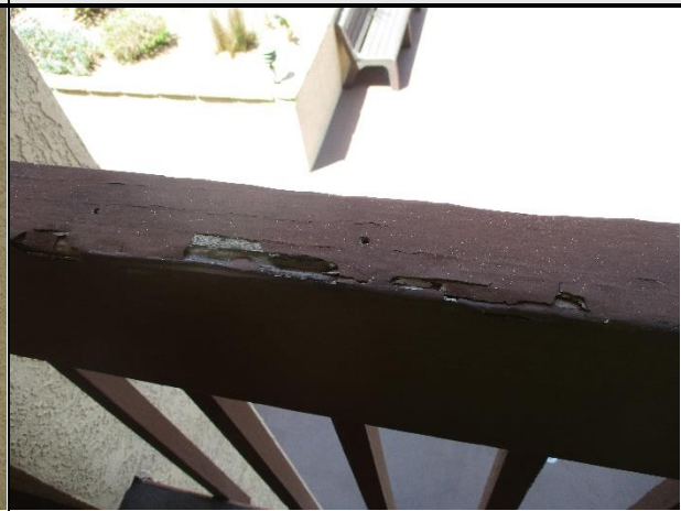
Handrail with Termite Damage
