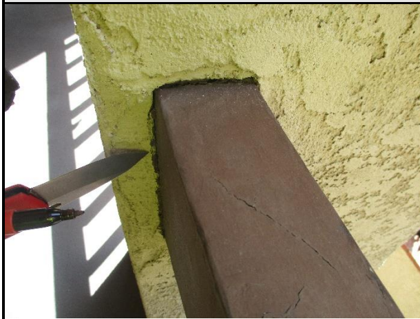
Typical Handrail with Poor End Flashing
