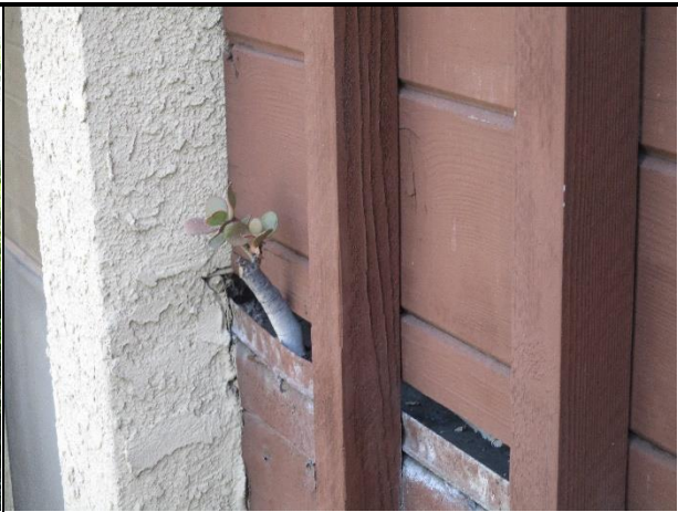
Plants Growing out of Flashing
