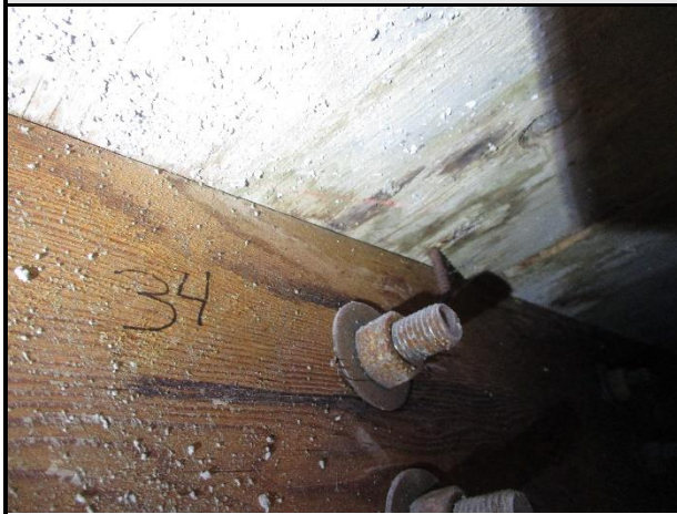
Corrosion on Bolts, Unbacked Fastener, Discoloration at Vent #34
