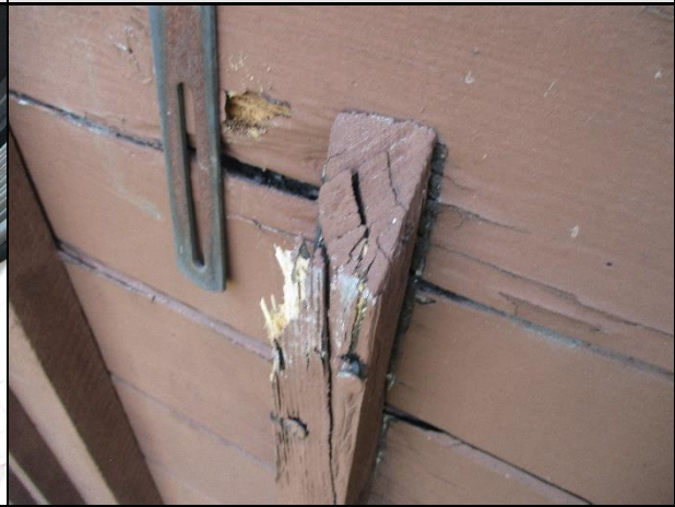
Termite Damage and Broken Picket
