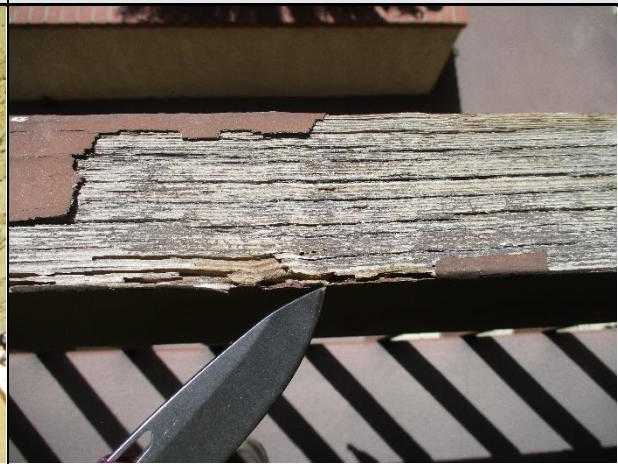
Handrail with Loss of Protective Coating and Termites
