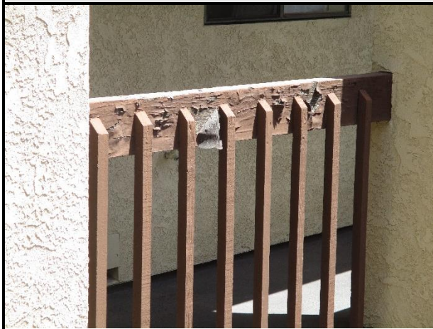
Typical Handrail Showing Deterioration
