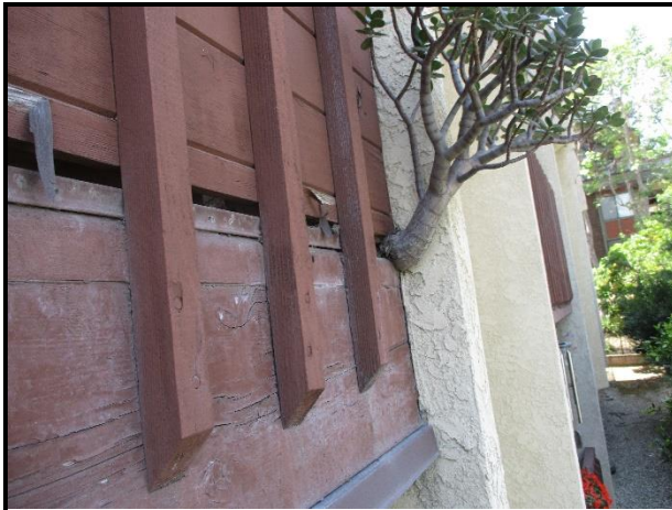
Plants Growing out of Flashing
